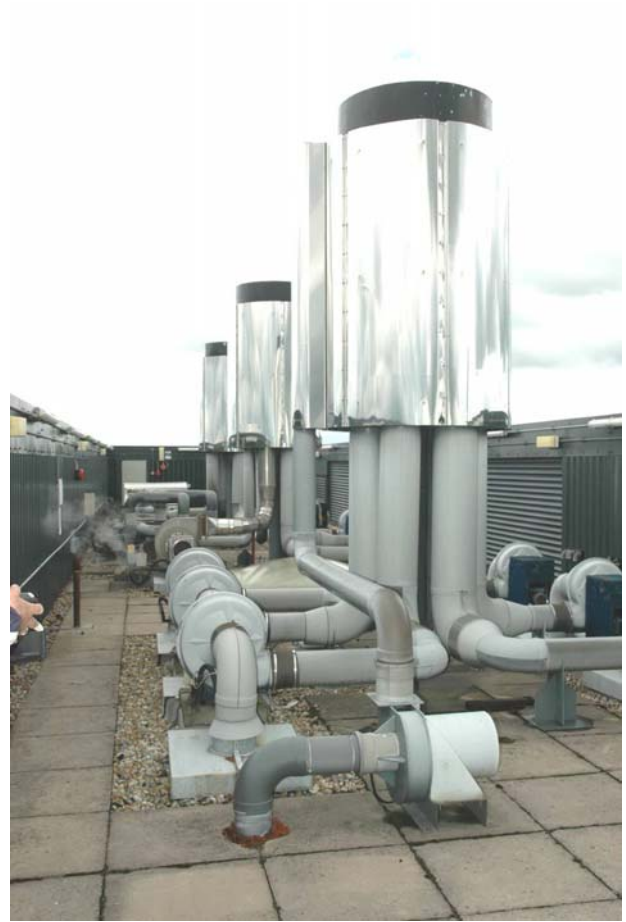
Extract fans and discharge stacks
