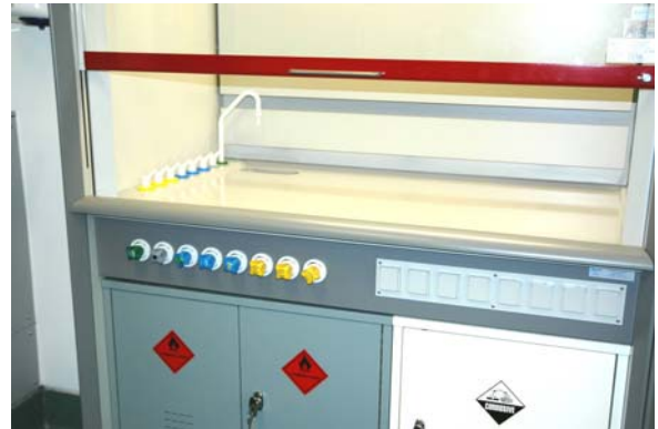
Fume Cupboard service outlets
