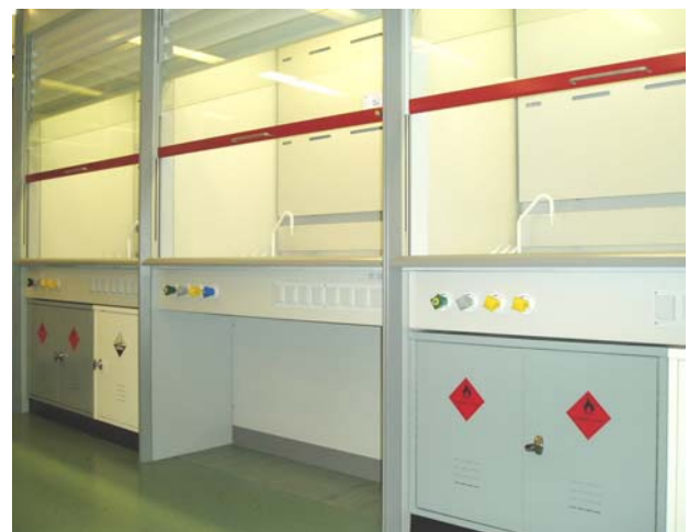
Low level storage
