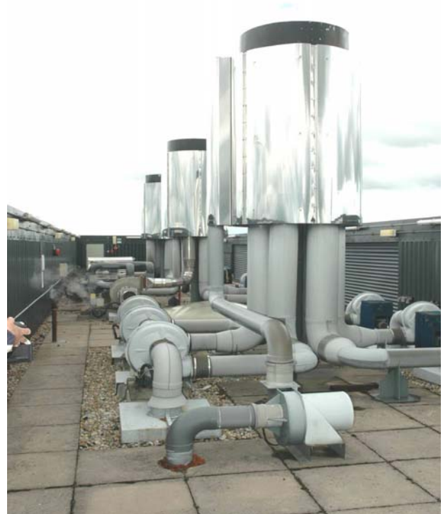
Extract fans and discharge stacks
